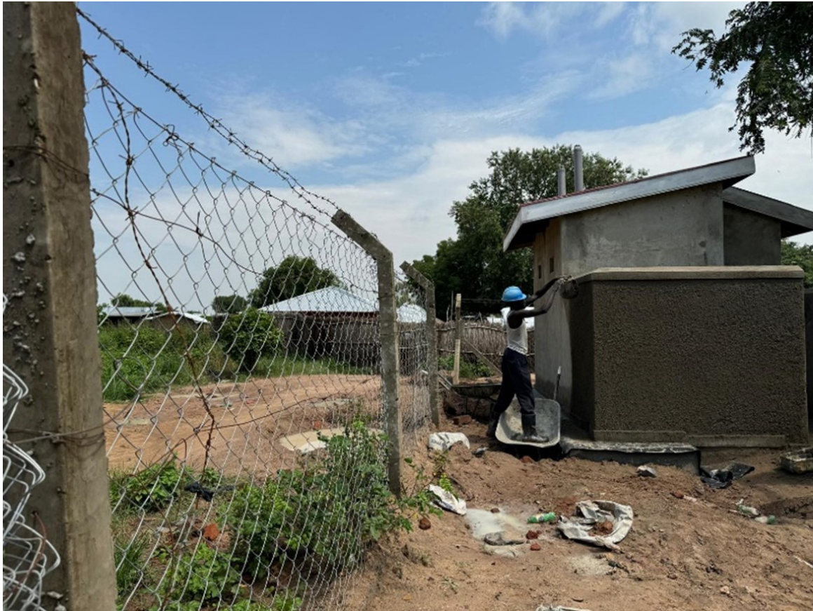
A latrine under construction in Rhino Camp's Ocea zone through a cash-for-work project. (Photo by USCRI Policy Analyst Daniel Salazar)
